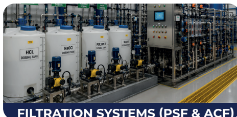
FILTRATION SYSTEMS (PSF & ACF)
