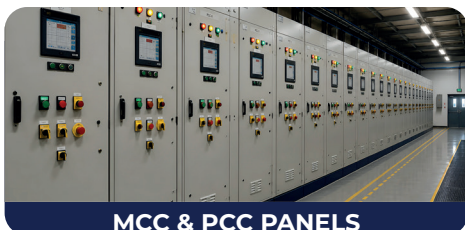
MCC & PCC PANELS
